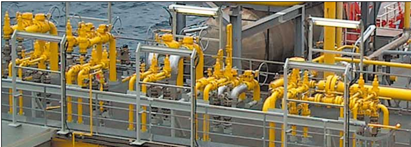
Typical offshore installation.
