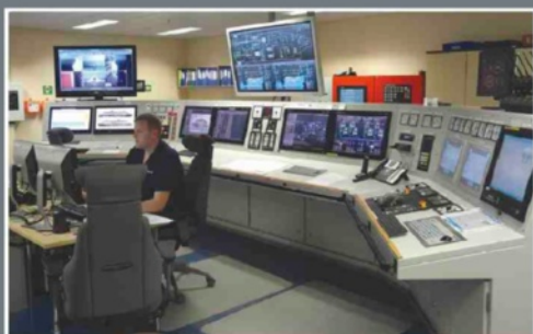
The engine control room.
