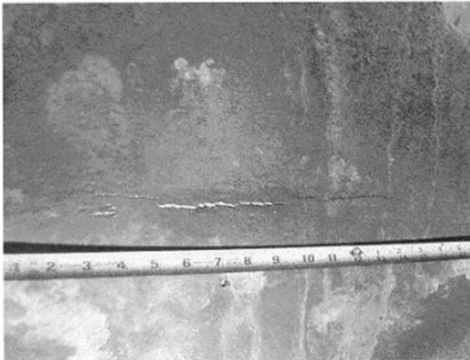
Fig. 4-13—Thermal fatigue cracking associated with bulged skirt shown in Figure 4-12.
