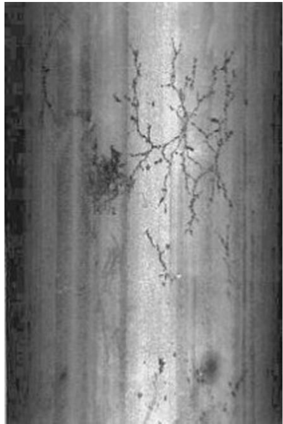
Fig. 4-79—Close-up of the tube in Figure 4-78 showing tight cracks with a spider web appearance.
