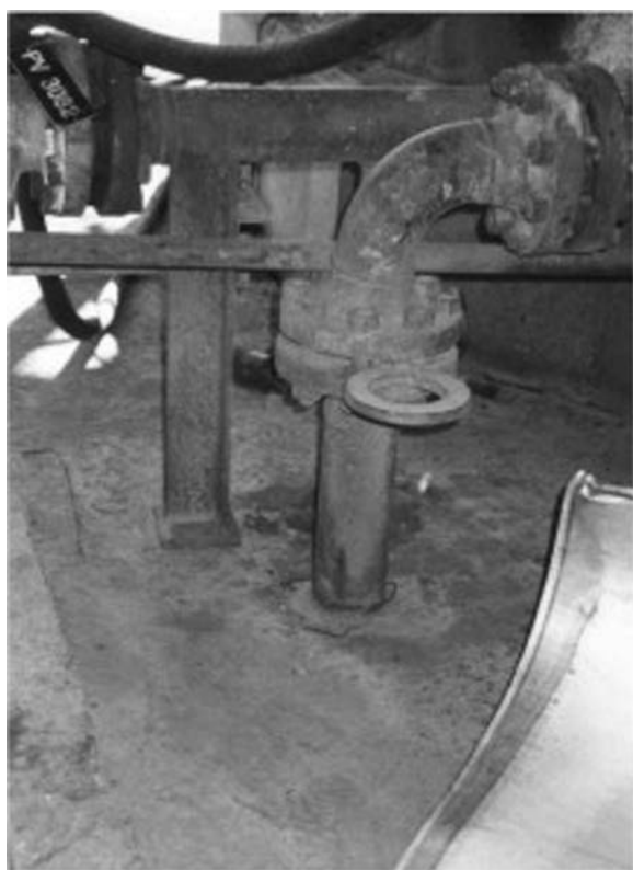
Fig. 4-51—Corrosion of carbon steel pipe at the soil-air interface where the pipe emerges from underground.
