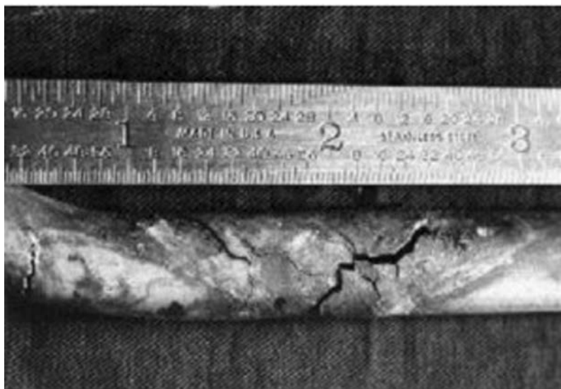
Fig. 4-77—External cracking of Type 304SS instrument tubing under insulation.
