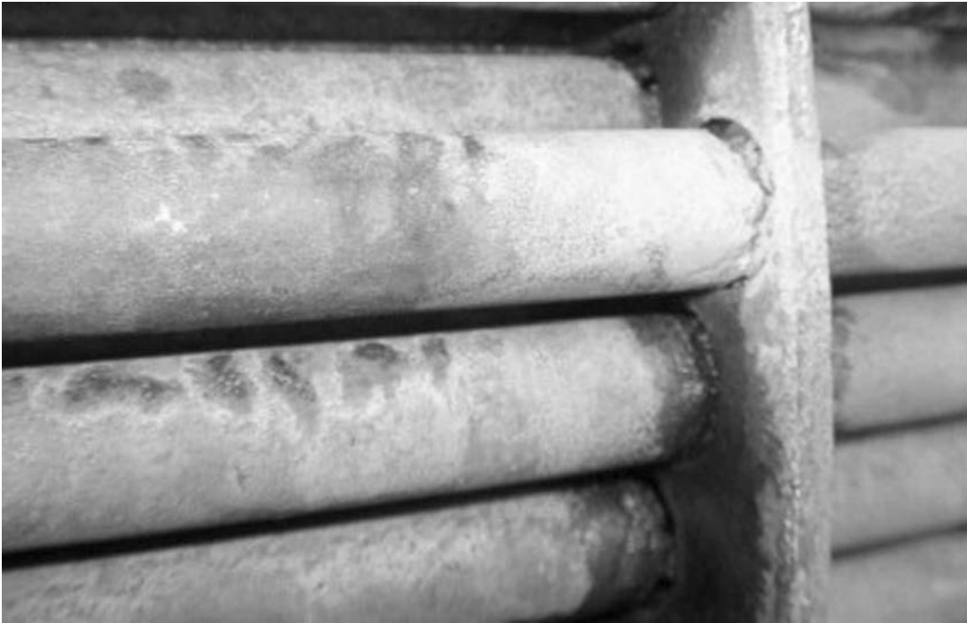
Fig. 5-9—Accelerated corrosion under a baffle.
