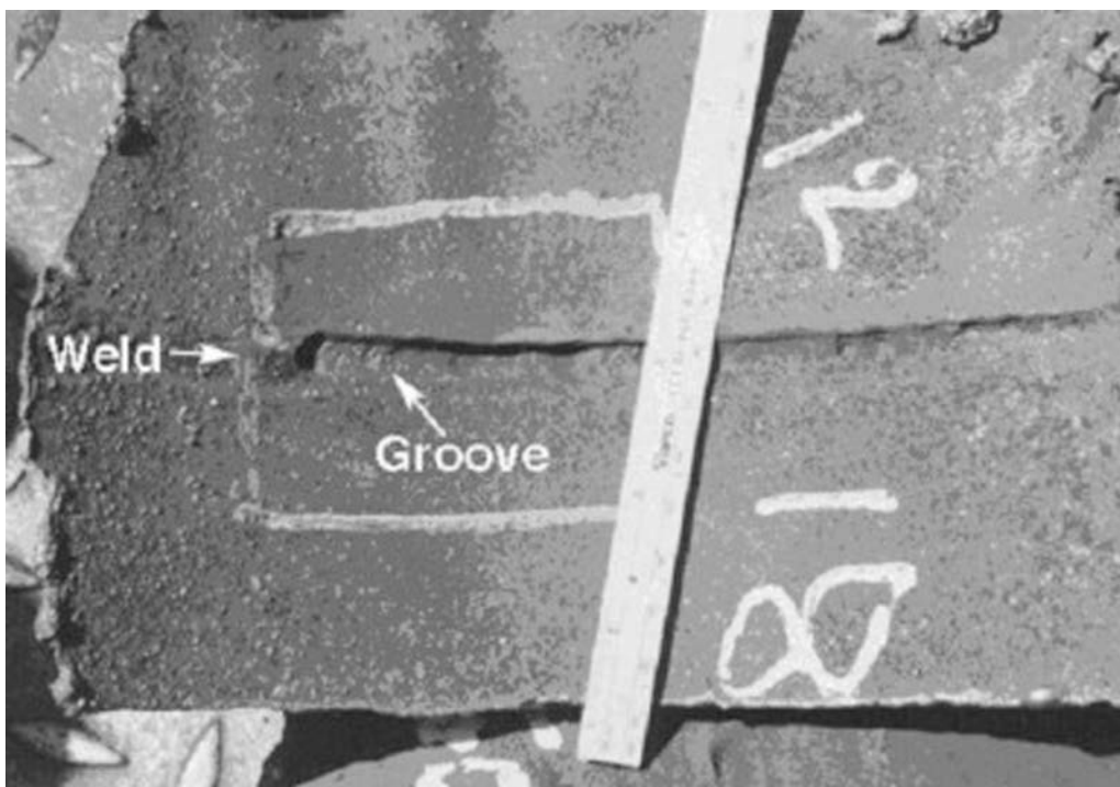
Fig. 5-1—Localized amine corrosion at the weld found in piping from reboiler to regenerator tower in an MEA unit. Many other similar cases found, some going as deep as half thickness. They were originally found and mistaken as cracks with shear wave UT inspection.
