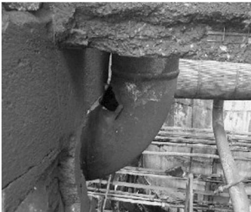
Fig. 4-67—Sulfidation failure of piping elbow.
