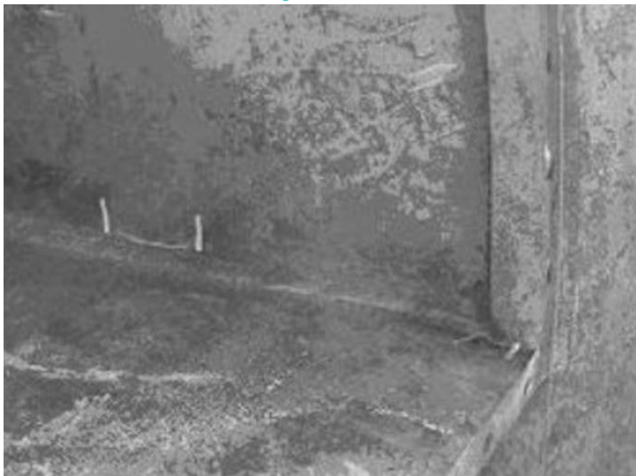
Fig. 4-99—Hydrogen embrittlement crack in a thick-wall 2.25Cr-1Mo exchanger channel circumferential weld. Hardness = 235 BHN
