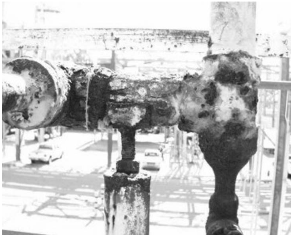
Fig. 4-38—CUI of CS level bridge
