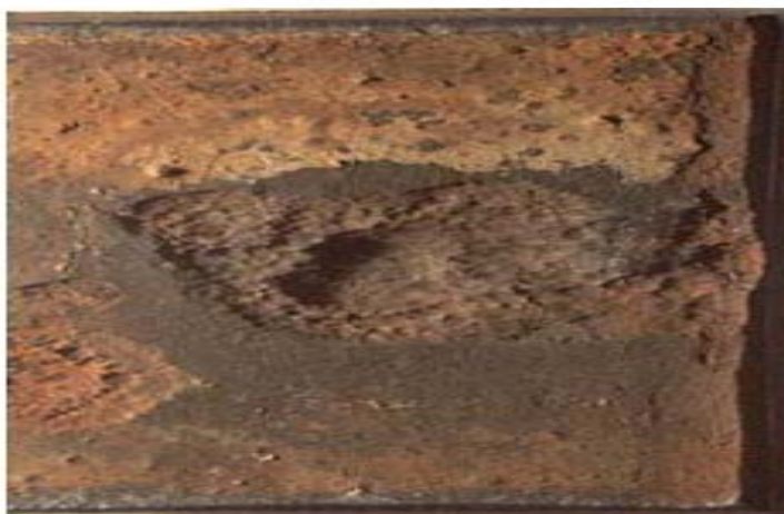
Figure 2.7 Corroded Carbon Steel Illustrating an Example of Pitting Corrosion
