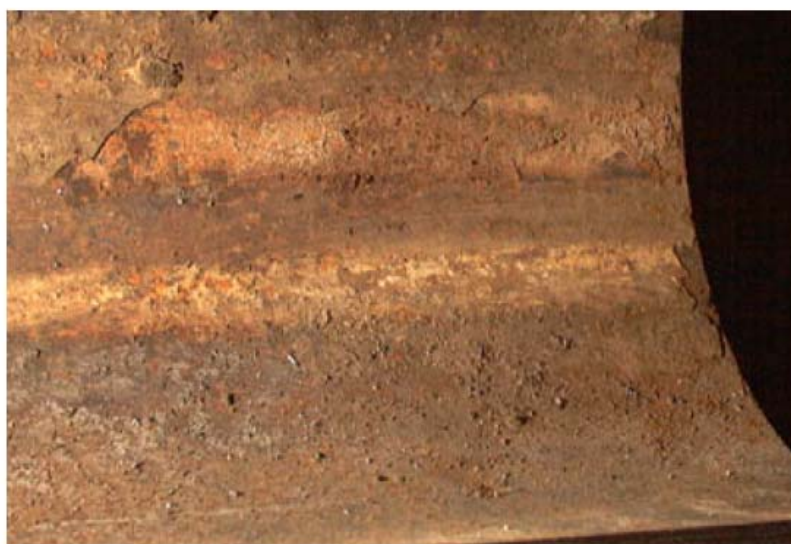
Figure 2.6 External Surface of a Pipeline With Uniform Corrosion
