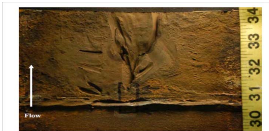
Figure 2.14 Grooves, Gullies, Waves, or Valleys Associated With Erosion-corrosion
