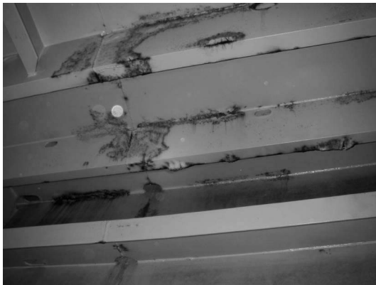
FIGURE 12.4 Corrosion creep initiating from welds and corners. (Photo: Børge Aune Schjelderupssen, Statoil.)
