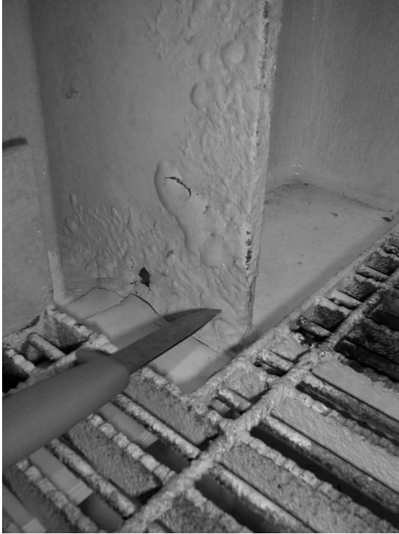
FIGURE 13.7 Corrosion of painted TSA. The TSA is corroding under the paint, causing the blistering of the paint.
