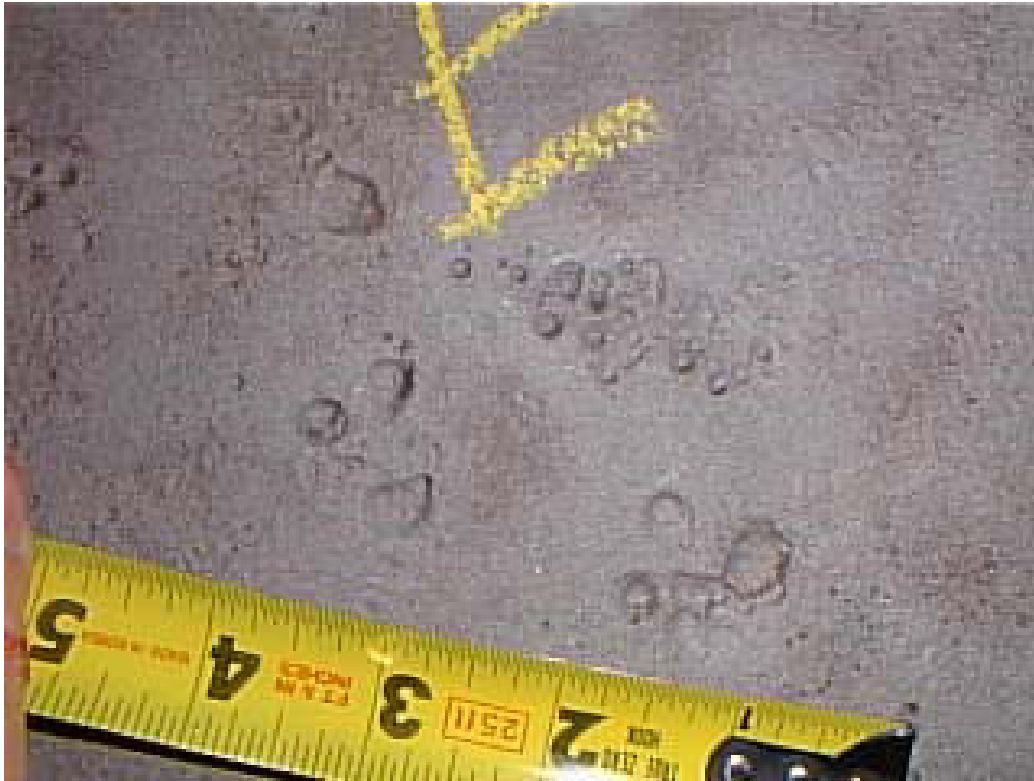
Figure E6.1-1 Example Problem E6.1 Pitting Damage
