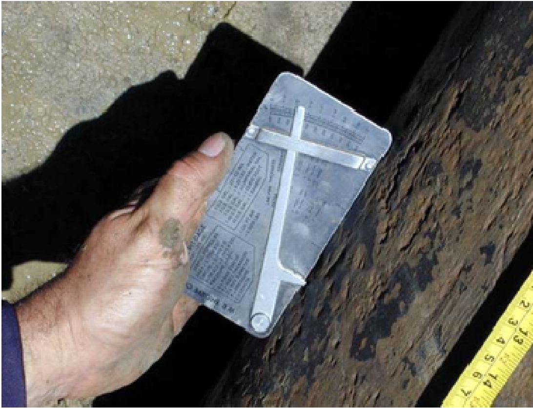
Figure E6.2-1 Example Problem E6.2 Pitting Damage
