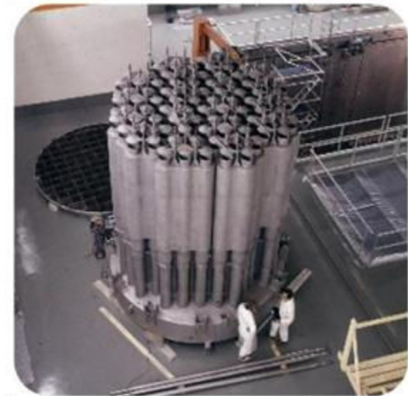
Steam separator, Oskarshamn Nuclear Power Plant
