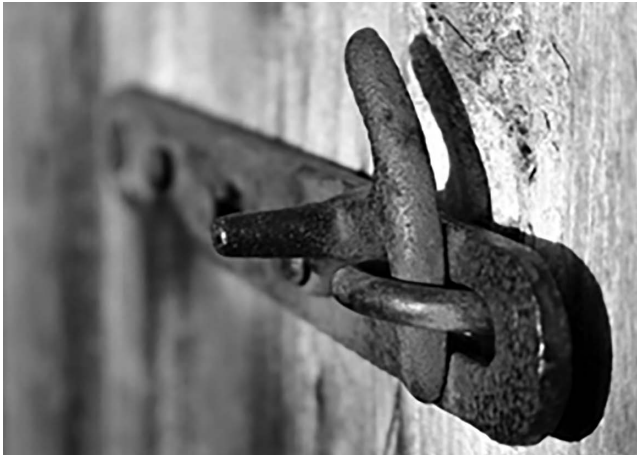
FIGURE 11.5 Galvanic corrosion in a wrought iron support system.
