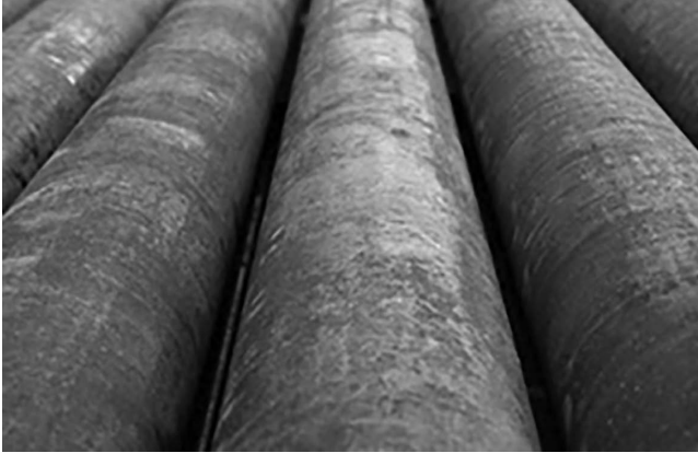
FIGURE 11.2 Uniform corrosion (rusting) of steel screw piles.
