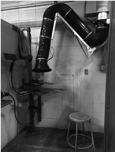
Figure I.13. Ventilation in a booth at NTC.
