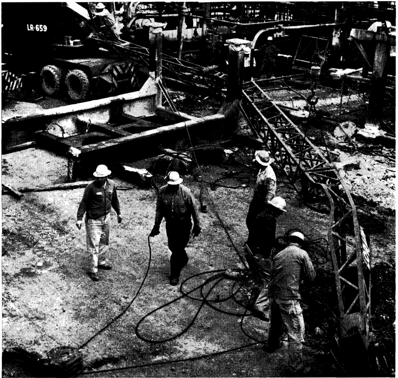
FIG. 50—In Dismantling Structure, Side Sway of Load Apparently Caused this Crane-Boom Failure.
