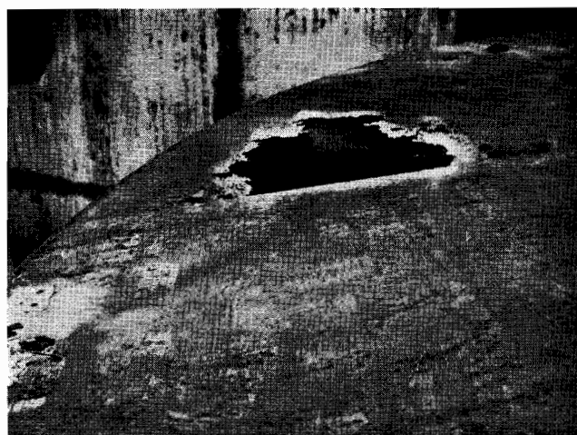
FIG. 13—A Severely Corroded Cone-Roof Tank Roof.
