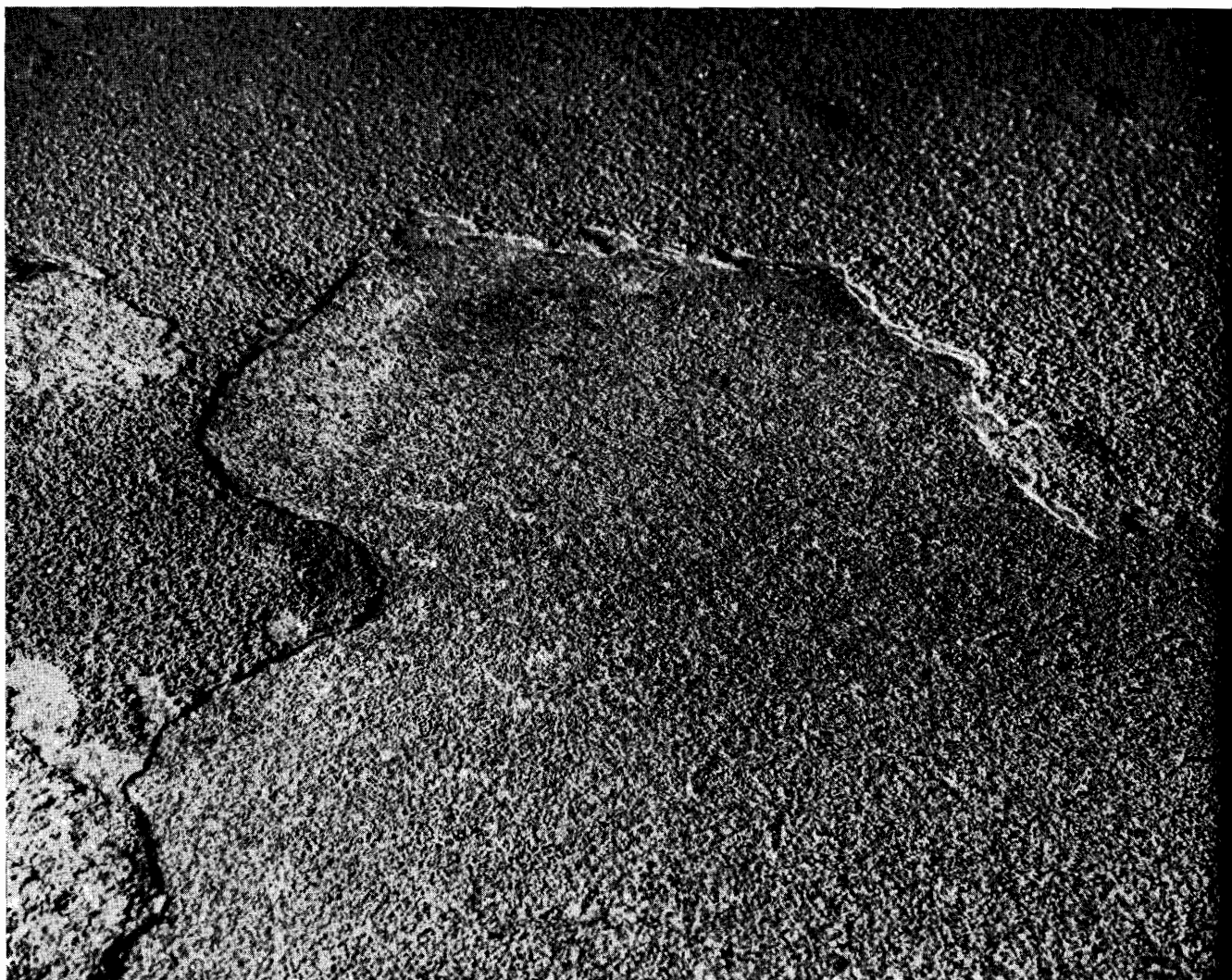
FIG. 18—Close-up of Corrosion on Underside of Floating-Roof Tank in Light-Stock Service.
