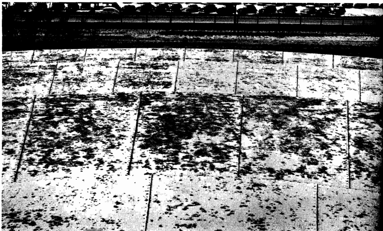
FIG. 24—Faulty Paint Job on this Tank Roof has Resulted in Accelerated Corrosion.
