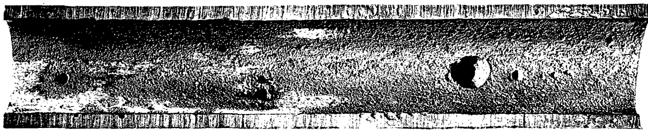
FIG. 23—Close-up of Phosphoric Acid Corrosion of a Carbon-Steel Reactor Feed Reactor Product Exchanger Tube in a Polymerization Unit.
