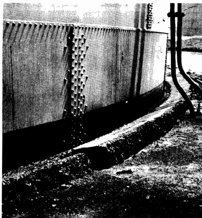
Figure 33—Failure of Concrete Base Ring
