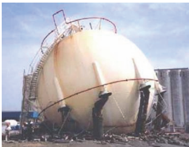
Figure 5—Failure of Sphere Legs Due to CUF
