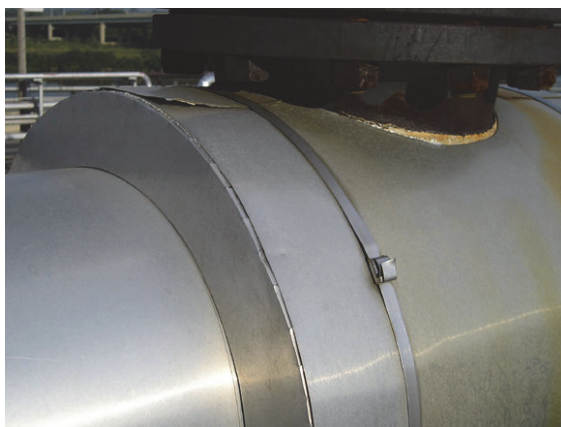
Figure 28—Example of Jacketing Joint with Missing Caulking
