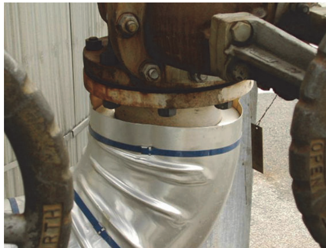
Figure 31—Example of Missing End Cap
