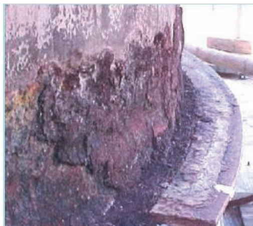
Figure 4—CUI at an Insulation Support Ring
