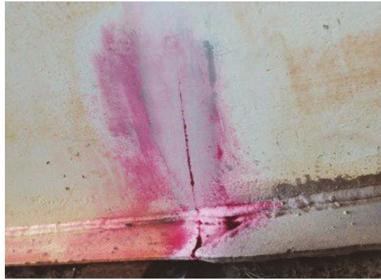
Figure 29—Cracks in Tank Shell Plate
