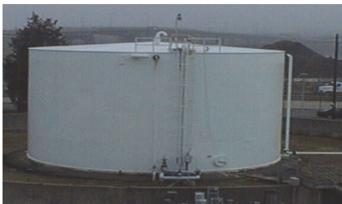
Figure 1—Cone Roof Tank
