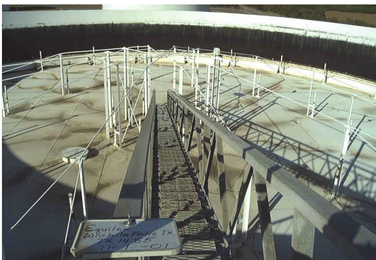
Figure 5—Pan Type Floating-roof Tank
