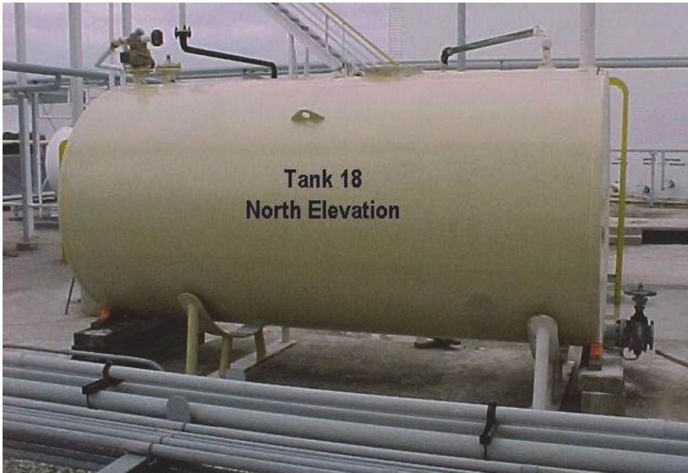
Figure 20—Welded Horizontal Tank Supported on Saddles
