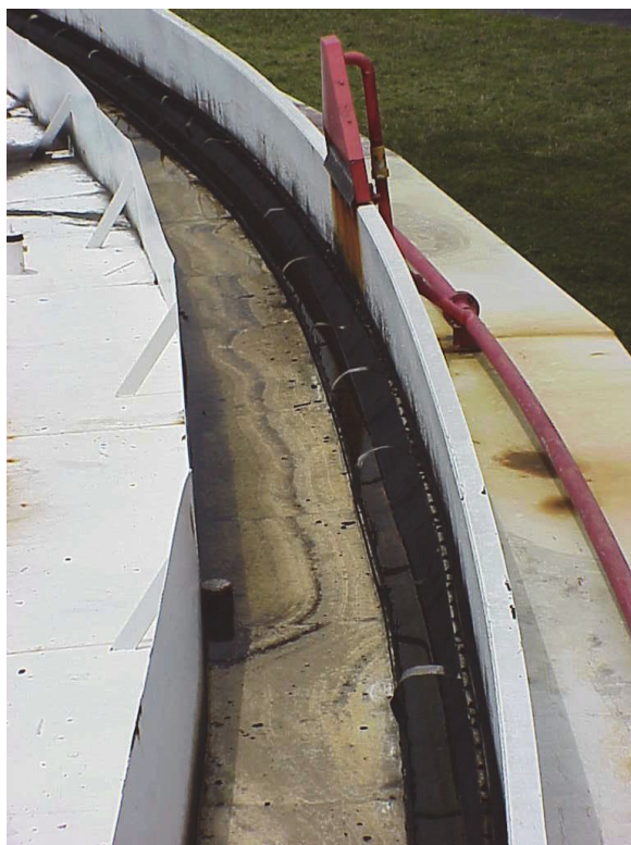
Figure 46—Deterioration of Floating-roof Seal
