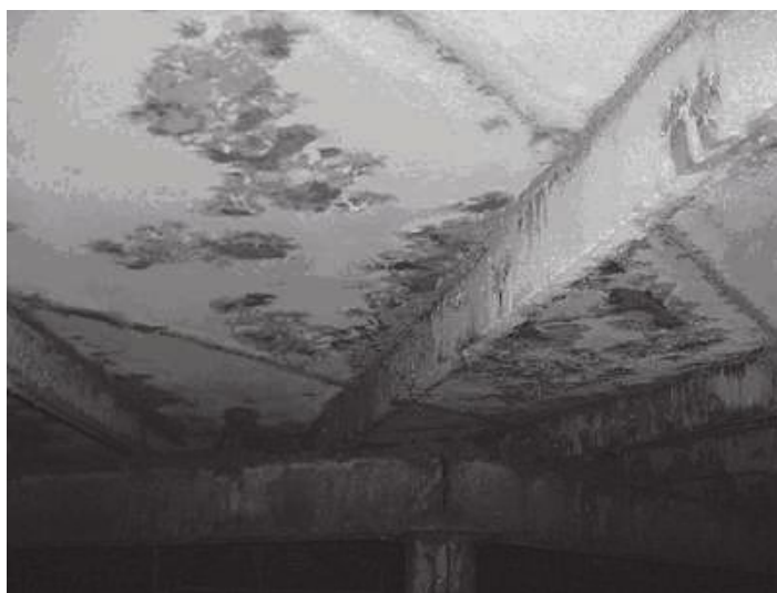
Figure 58—Internal Corrosion on Rafters and Roof Plates
