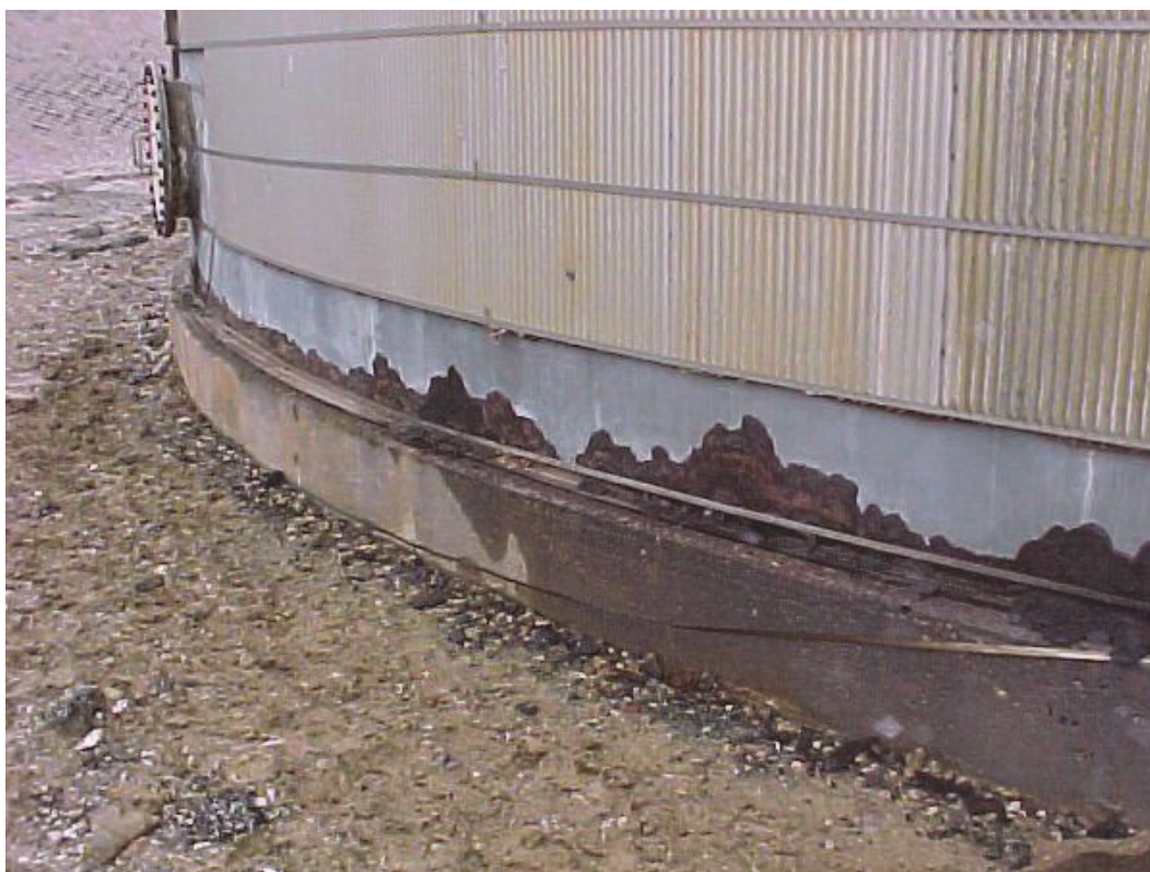
Figure 37—Corrosion Under Insulation
