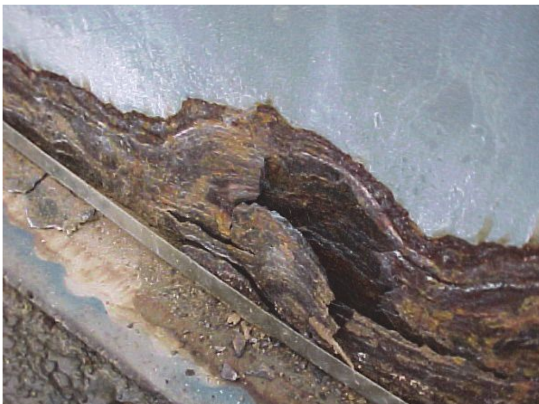
Figure 38—Close-up of Corrosion Under Insulation
