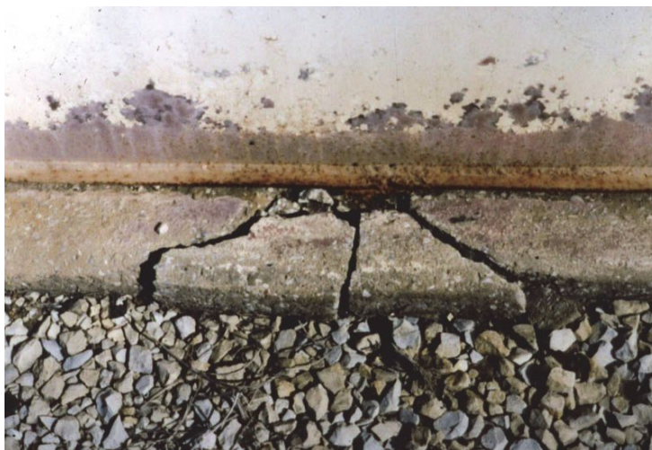
Figure 34—Failure of Concrete Ringwall
