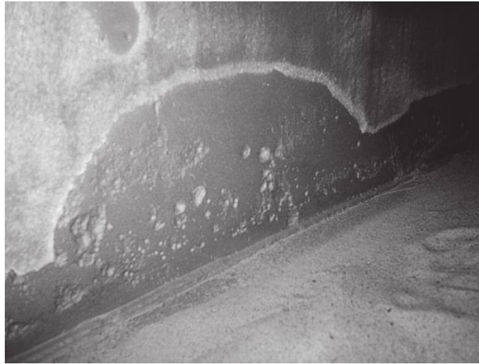
Figure 55—Shell-to-bottom Weld Corrosion
