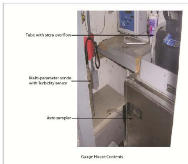
FIG. 19 Contents of gage house showing sonde and sidestream vessel
