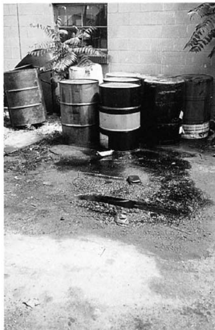
FIG. X1.12 Surface Staining from Improper Drum Storage
