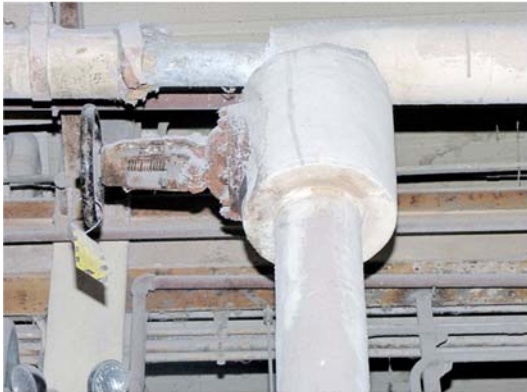
(h) Valve and Piping Insulation P2
