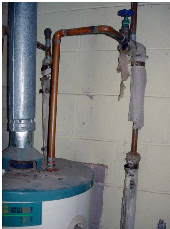
(b) Pipe Insulation in Mechanical Room
