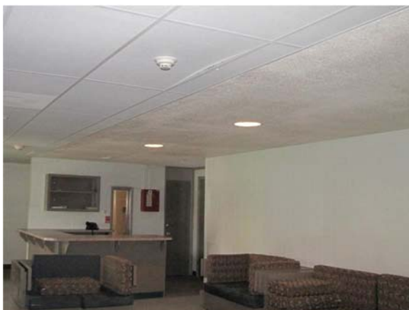
(c) Textured Ceiling Finish in Lobby C3
