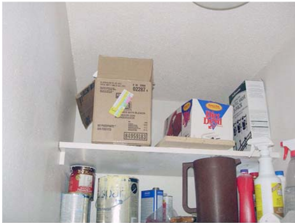
(b) Closet Ceiling Plaster C2
