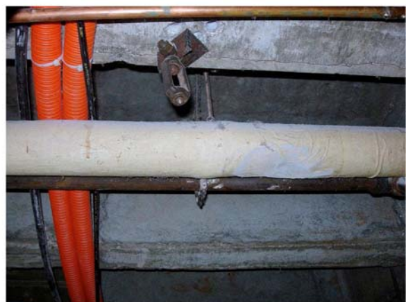
(f) Mechanical Room Pipe hanger P1
