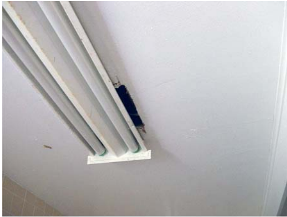
(a) Restroom Ceiling Plaster C1
