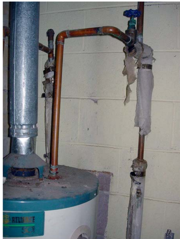
(b) Pipe Insulation in Mechanical Room
