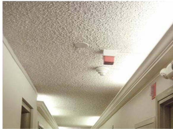
(e) Hallway Ceiling Plaster C5
