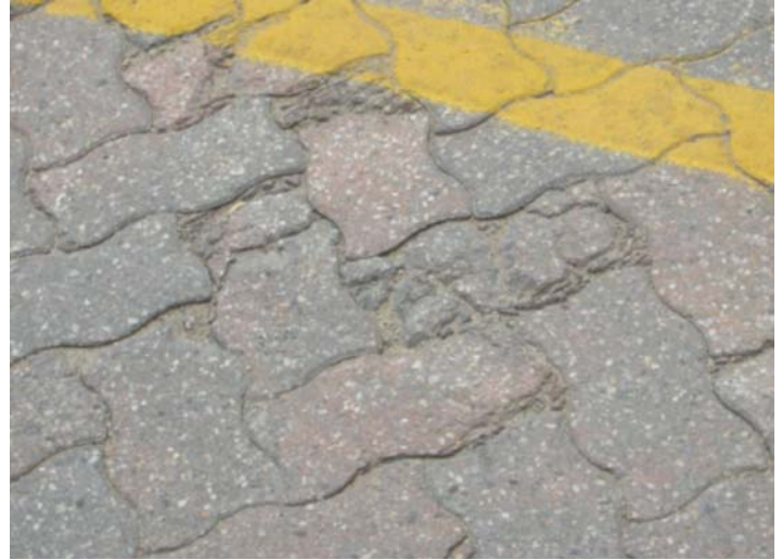
FIG. X1.2 Medium Severity Damaged Pavers
