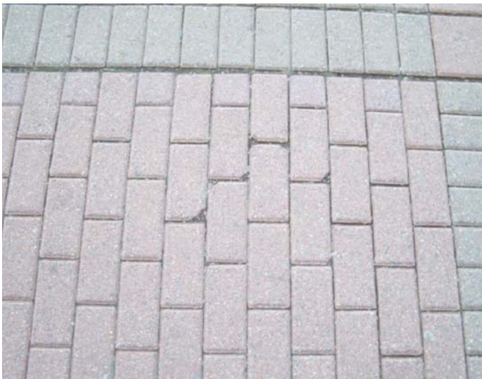
FIG. X1.1 Low Severity Damaged Pavers
