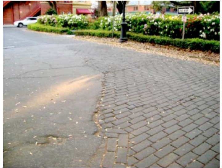
FIG. X1.29 Medium Severity Patch
