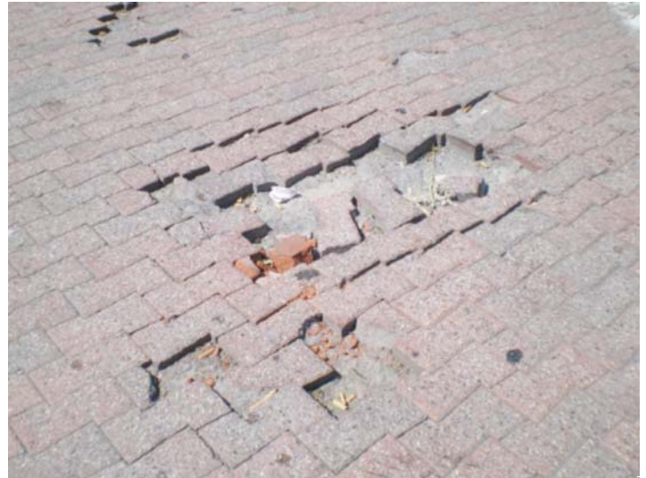
FIG. X1.27 High Severity Missing Pavers
