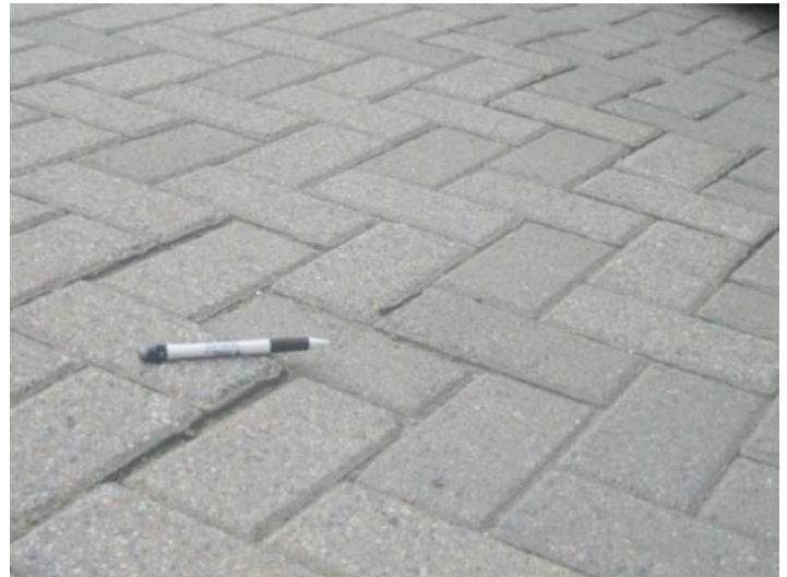
FIG. X1.15 High Severity Faulting
