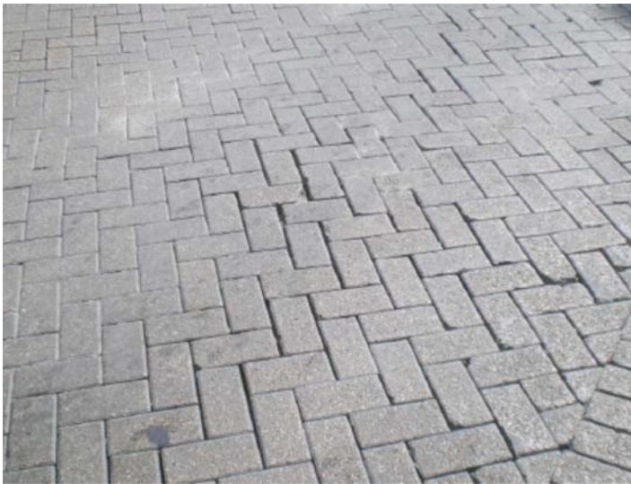
FIG. X1.19 Low Severity Horizontal Creep
