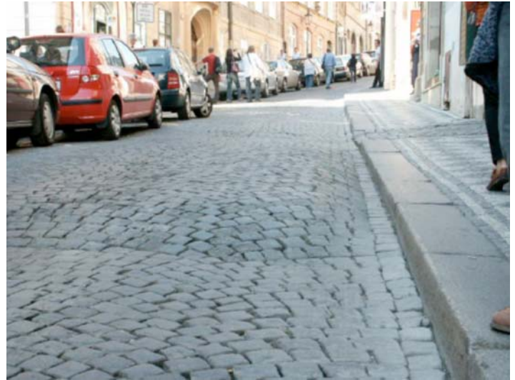
FIG. X1.18 High Severity Heave
