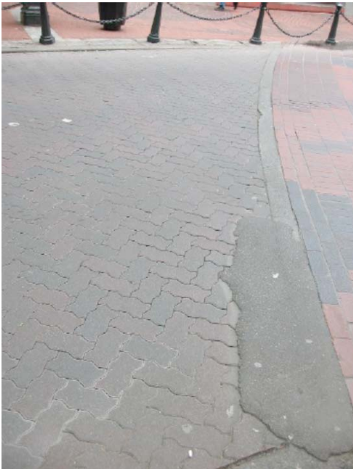
FIG. X1.28 Low Severity Patch
