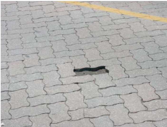
FIG. X1.25 Low Severity Missing Pavers
