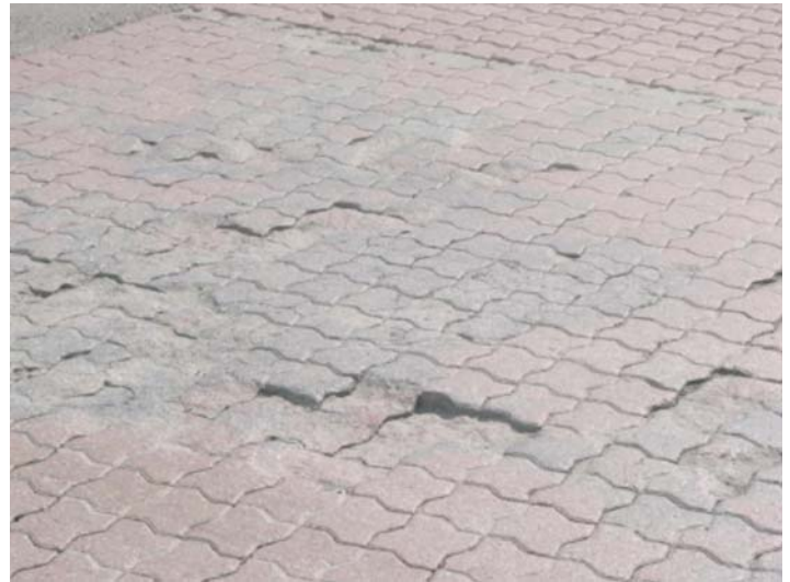
FIG. X1.3 High Severity Damaged Pavers
