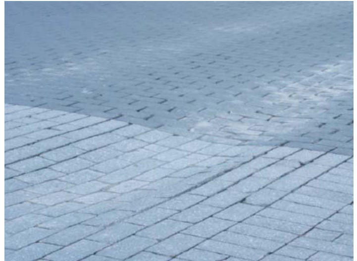
FIG. X1.32 Medium Severity Rutting
