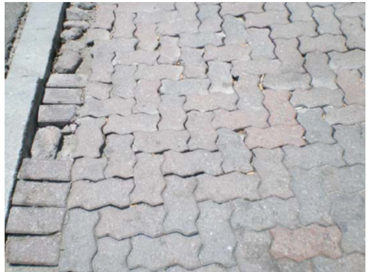
FIG. X1.9 Medium Severity Loss of Edge Restraint
