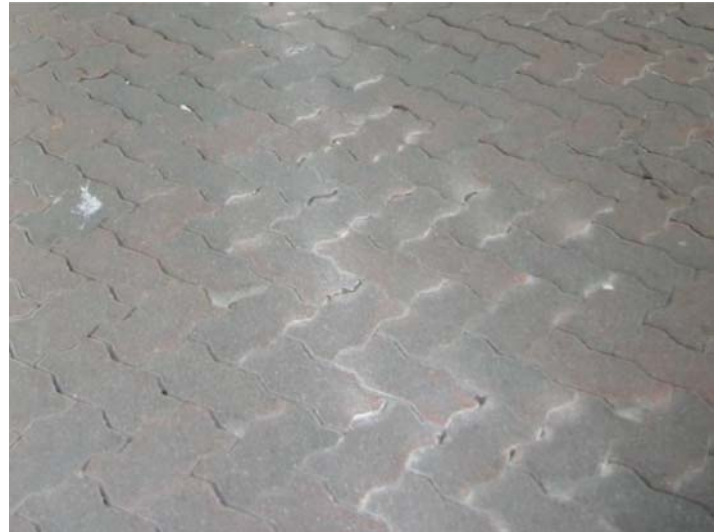
FIG. X1.23 Medium Severity Joint Sand Loss
