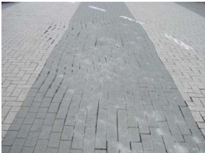
FIG. X1.7 High Severity Loss of Edge Restraint
