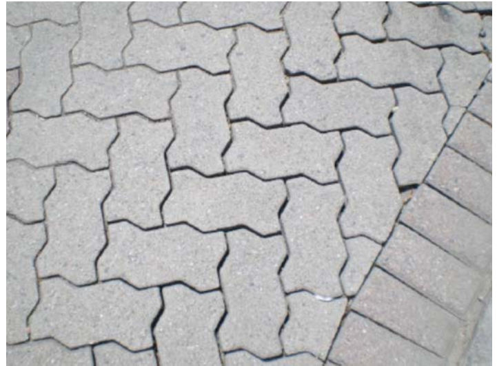
FIG. X1.11 Medium Severity Excessive Joint Width
