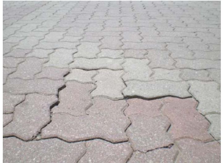
FIG. X1.14 Medium Severity Faulting
