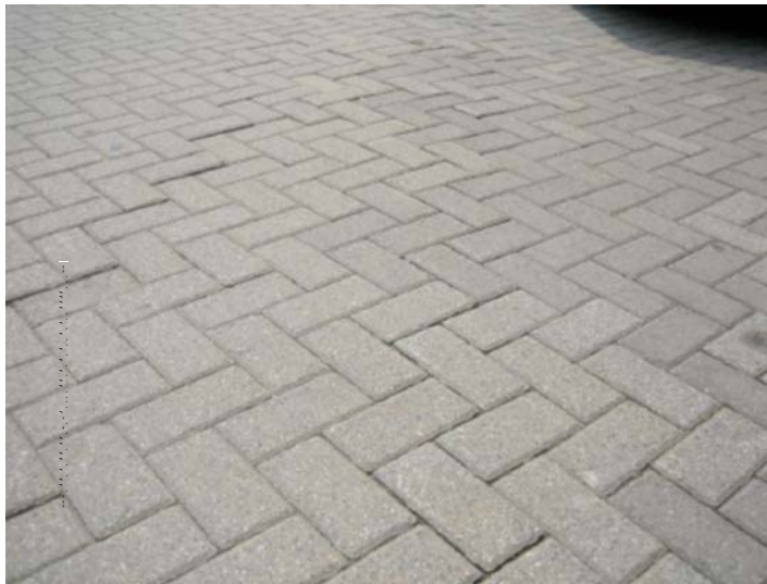
FIG. X1.13 Low Severity Faulting
