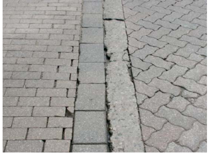
FIG. X1.8 Low Severity Loss of Edge Restraint
