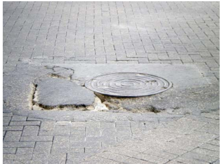
FIG. X1.30 High Severity Patch
