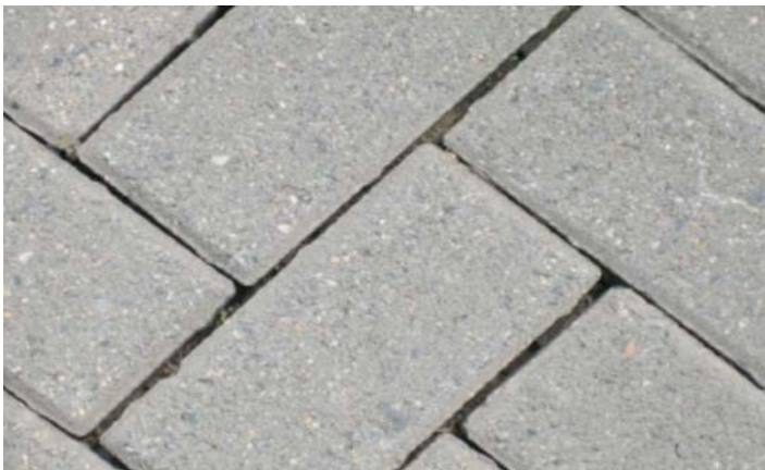
FIG. X1.22 Low Severity Joint Sand Loss
