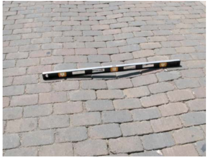
FIG. X1.33 High Severity Rutting
