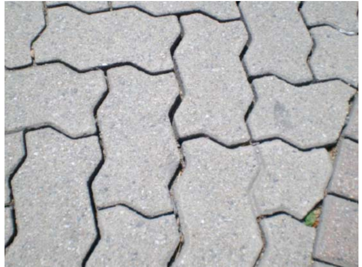
FIG. X1.24 High Severity Joint Sand Loss
