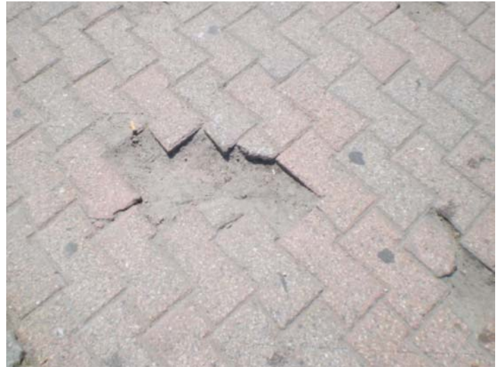
FIG. X1.26 Medium Severity Missing Pavers
