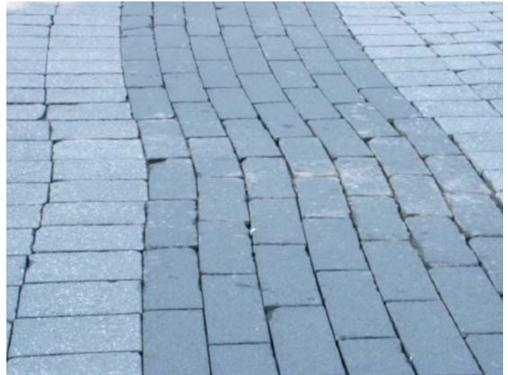
FIG. X1.21 High Severity Horizontal Creep
