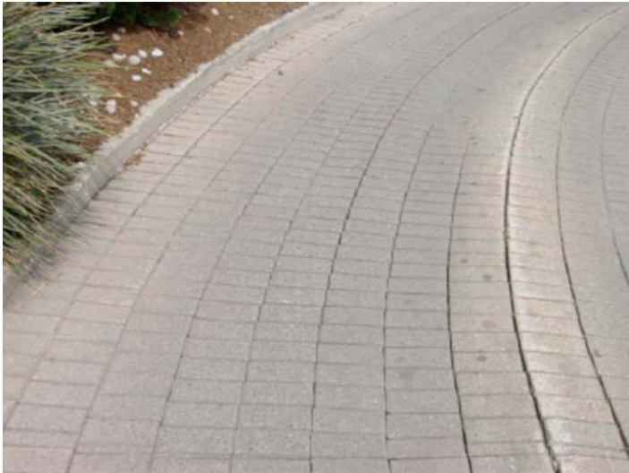
FIG. X1.31 Low Severity Rutting
