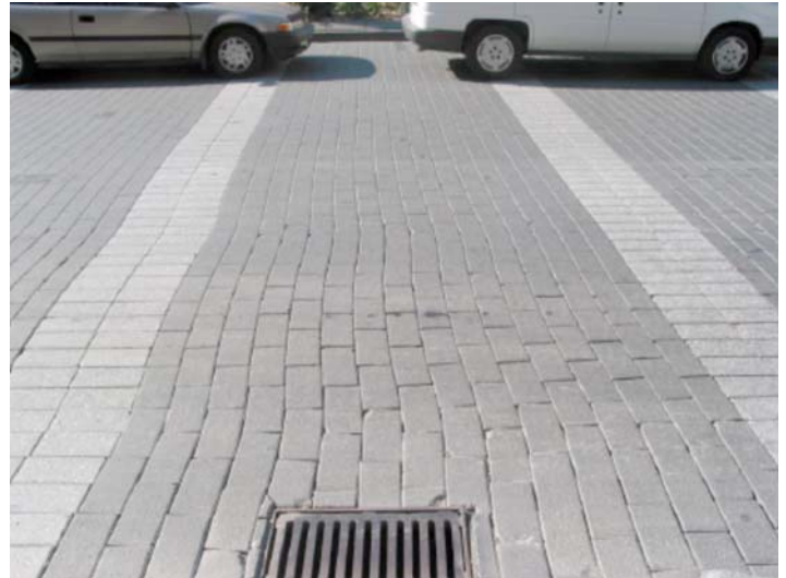
FIG. X1.20 Medium Severity Horizontal Creep
