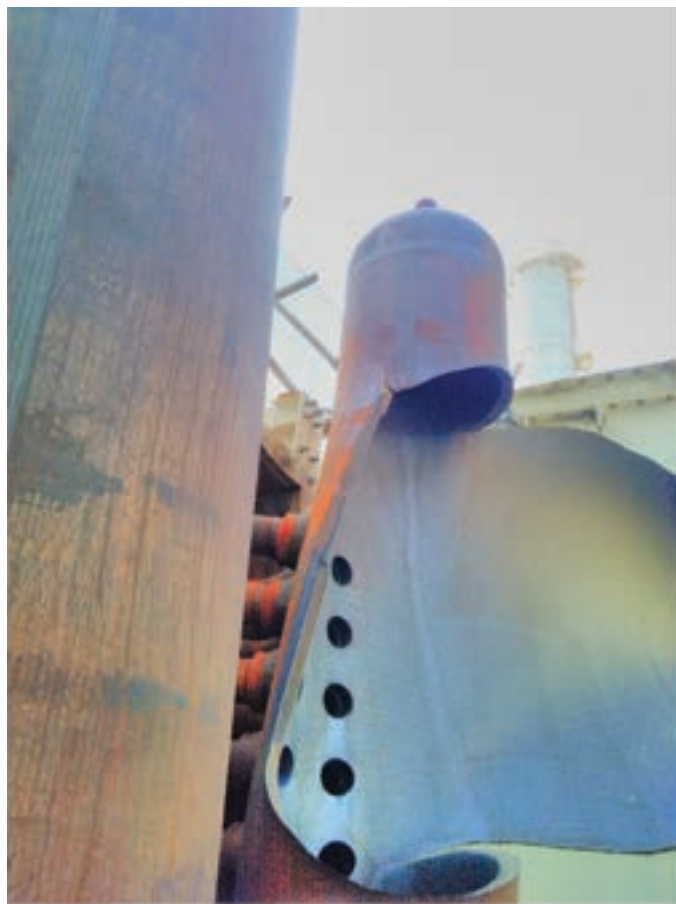
Figure 1. Ruptured superheated steam outlet header.
