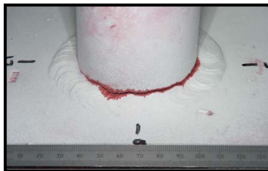
Figure 11 Crack found using Dye-Penetrant Inspection
