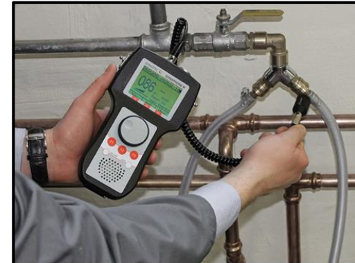
Ultrasonic Leak Detection
