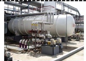
Pressure Vessel System
