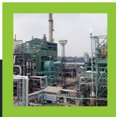
Unfired Steam Generators (boilers)
