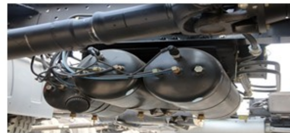
Air receivers associated with braking systems of mobile equipment
