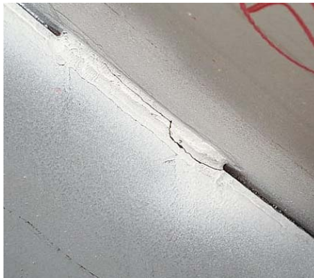
Crack found using magnetic particle inspection.
