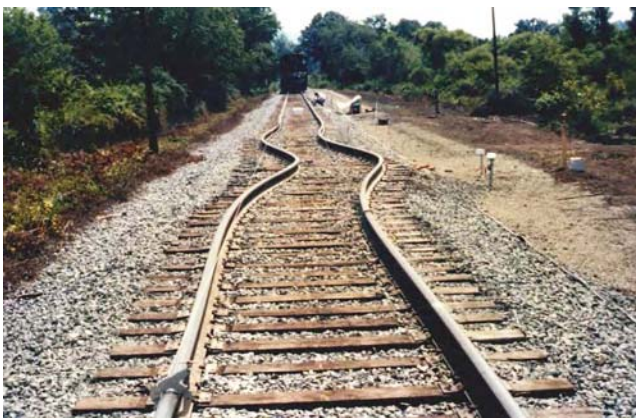
Figure 4.2 Photograph showing buckling of the steel rails of a railroad track because of thermal expansion under unusually high atmospheric temperatures. Some dramatic examples of the so-called “rail buckling” can be viewed in YouTube. Source: Photograph by the US Department of Transportation and in the public domain for free use.
