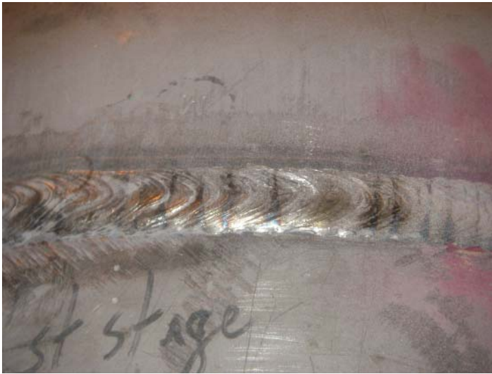
Figure 6.5 Photomicrograph showing transverse cracks in a circumferential weld made in steel. Source: website www.ndt.net , appearing in a response to a question from Juan Amado by Deston Henson, NDT Inspector of Canada, on 21 January 2011. Used with kind permission of Deston Henson.
