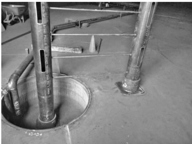
Ladder, slotted gauge pole, and sump.
