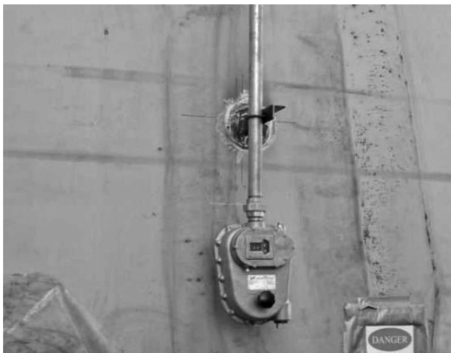
Gauging system (mounted exterior).
