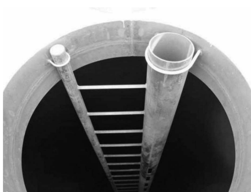
Internal ladder with slotted gauge pole.
