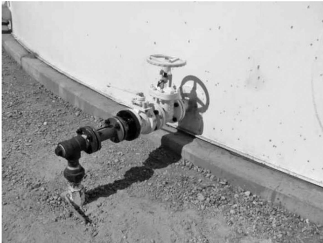
Water draw off piping.
