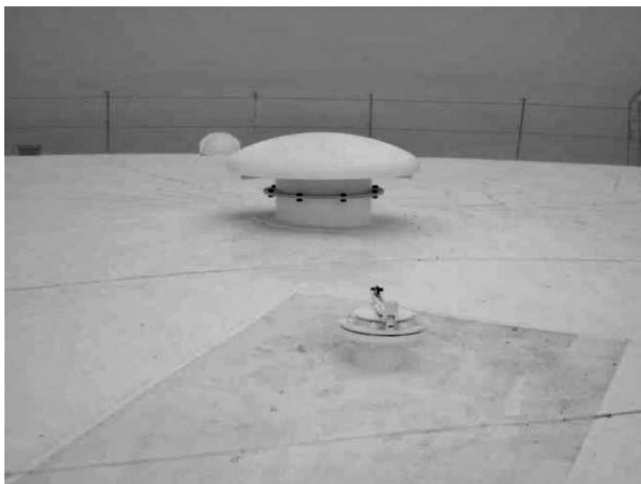
Fixed roof mushroom circulation vent.
