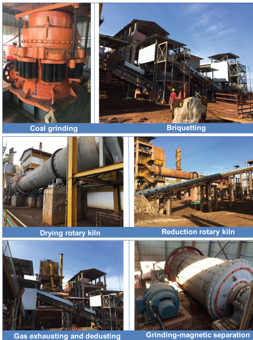
Fig. 2.66 Main facilities for the new process of preparing ferronickel through coal-based rotary kiln direct reduction-magnetic separation
