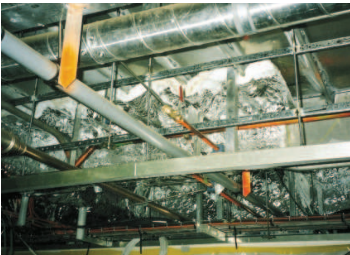
INSULATION IN THE ENGINE ROOM
