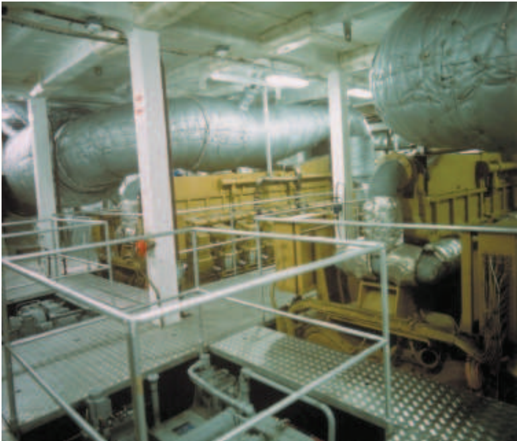
ENGINE ROOM OF THE AQUASTRADA TMV 115
