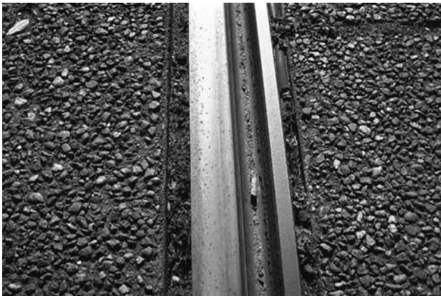
FIGURE 5.3 Pitting on a frequently used tram track.
