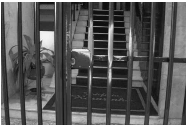
FIGURE 8.5 Tribocorrosion of an entry gate (anodized coating on aluminum) from rubbing produced by user's hands.
