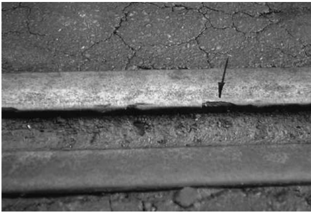
FIGURE 5.2 Rolling contact fatigue on a railroad track that produced spalling.
