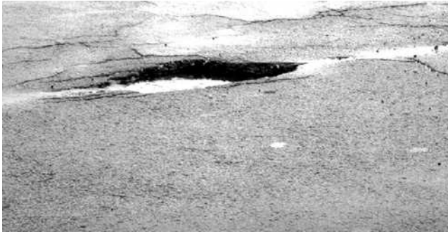
FIGURE 5.1 Rolling contact fatigue of a macadam roadway.
