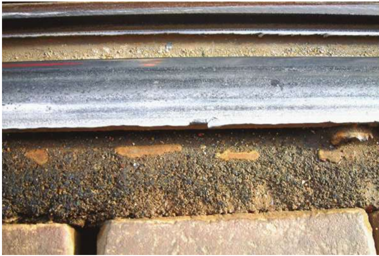
COLOR FIGURE 5.5 Cracking on a railroad track.
