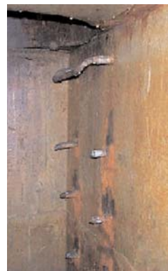
Corroded ladder rungs
