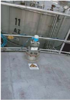
Level gauge on top of tank
