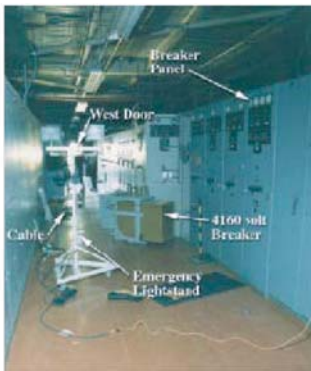
Switchgear looking towards the exit door
