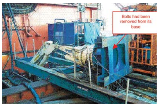
Toppled SIMOPS crane
