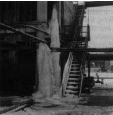
Figure 14 Freezing water leaks create hazardous working conditions.
