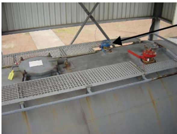
Valve which was due for repairs.
