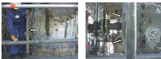
The deformed / bulged section of the overheated reactor from a runaway reaction.
