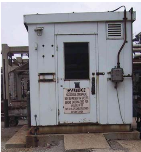
Analyser house with atmosphere warning signs.
