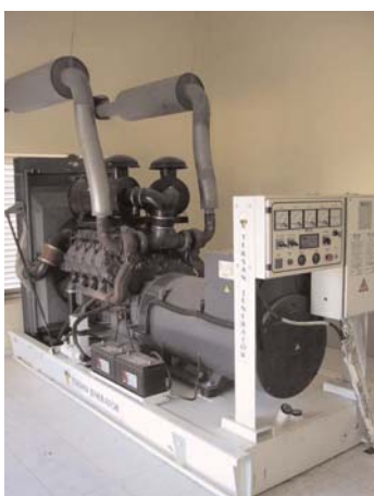
Diesel electricity generator
