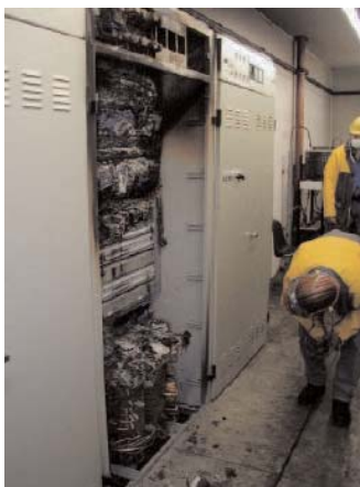
Extent of damage to cabinet.
