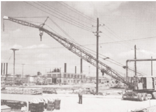
Figure 67 Someone should have the primary duty of directing crane operation near overhead electrical lines.
