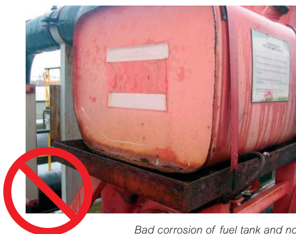
Bad corrosion of fuel tank and no secondary containment for the full capacity
