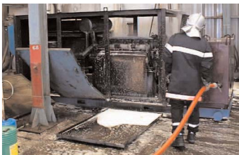
Diesel generator destroyed by fire in a BP facility.
