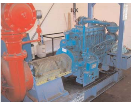
Diesel fire pump
