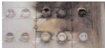
Burnt electrical panel.
