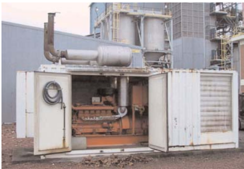
Typical diesel driven emergency generator installed as a skid in a container to supply emergency power to a chemical plant.
