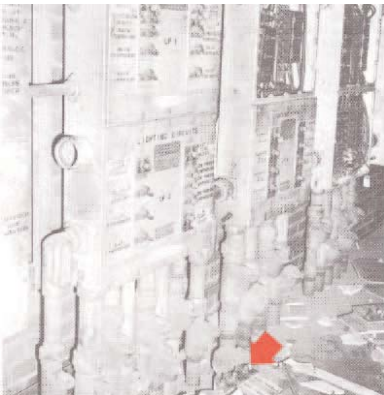
Figure 51 Gas entered vapourtight lighting panelboard housing through underground conduits and exploded when a panelboard switch was operated.
