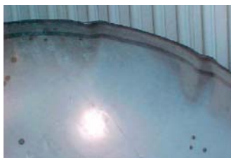
Damaged tank compartment joint
