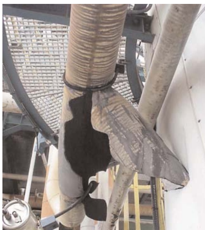
Pipe ruptured due to overpressure.
