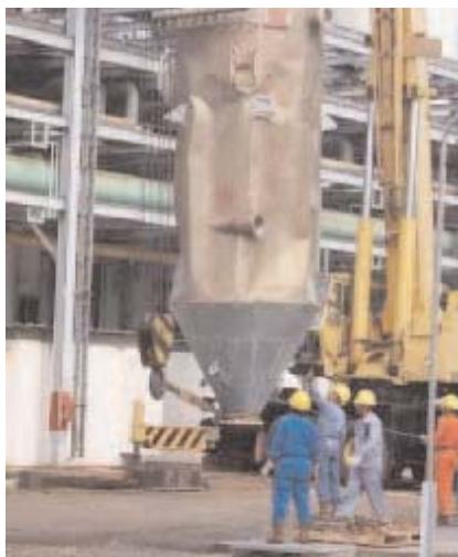
Damaged cyclofilter being removed for repairs.
