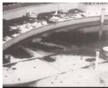
Example of a roof with waxy deposits
