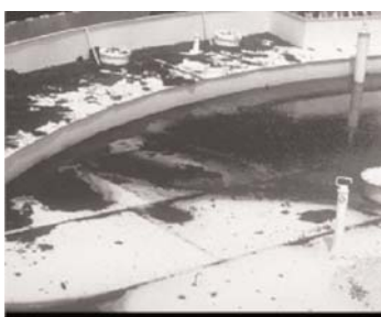
Example of a roof with waxy deposits
