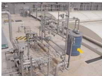
Good example of closed API separator with carbon canister absorbing system to prevent VOC emissions to atmosphere (Refer to Section 9.7 for the hazards of carbon canisters).
