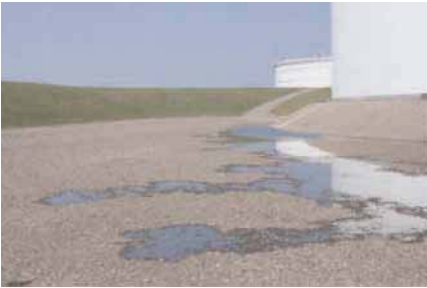
Oil spill from leaking roof drain
