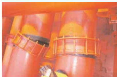
Damage to ship's 24-inch (600 mm) pipework in way of expansion couplings
