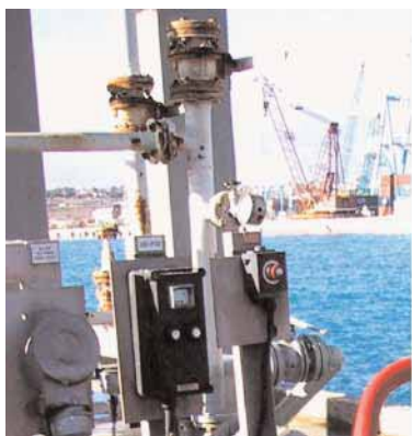
Difficult to see the ESD button and no indication of what is shut down.
