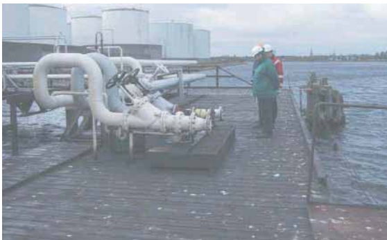
Wooden jetty with gaps between planks—no retention against spills
