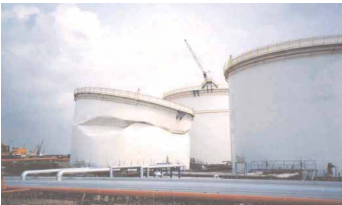
Failed/buckled tank shell due to excessive internal corrosion
