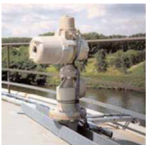
Level gauge on a tank roof
