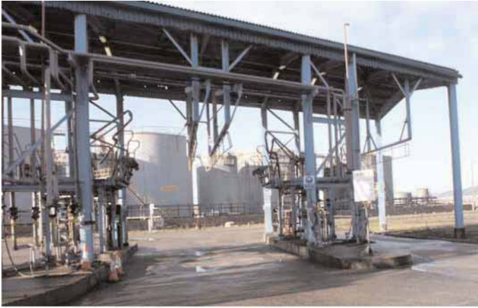
Road tanker loading racks
