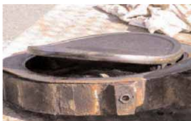
Damage to Marine Arm's 16-inch (400 mm) butterfly valve
