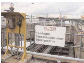
Good example of API separator with skimmer tilt controls extended out of the pit so that operators do not have to go into the pit. It also has good signage, and gas detection with a visual alarm.
