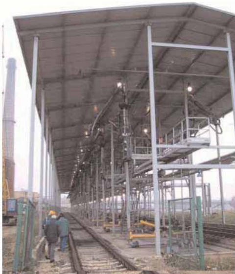
Rail tanker loading racks
