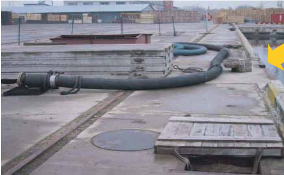
Missing sections of retention wall to prevent spill from hose entering the sea.
