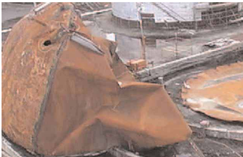
Spent acid tank explosion separating roof and shell from the bottom plate
