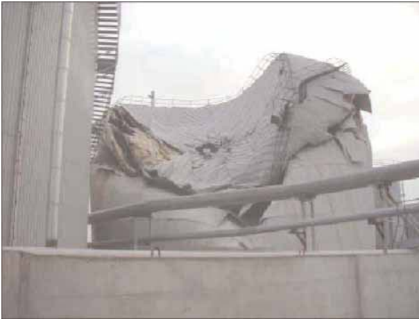
Tank collapsed due to rustiness and severe gale
