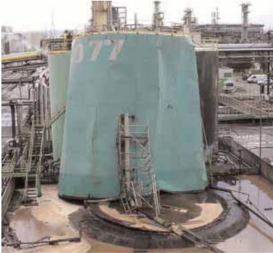
Shell to bottom weld rupture (tank overpressured when purging a line with nitrogen)
