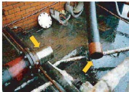
Close up of failed compression joint
