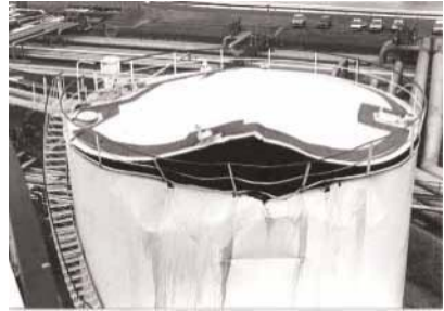
Shell to roof weld rupture
