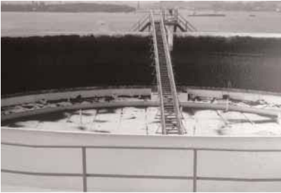
Rust and debris on floating roof can block the internal drain
