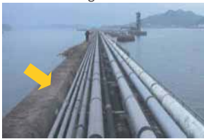
Unsafe access to jetty
