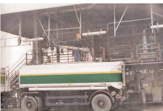
Top loading of a road tanker using a loading arm
