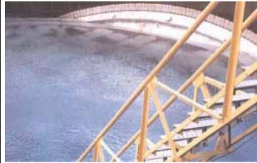
Sunken floating roof due to accumulation of rainwater on the roof
