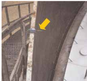
Independent high level alarm on a floating roof tank
