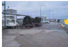
No safety rail to prevent vehicles falling off jetty
