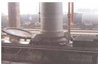
Loading and vapour recovery arrangement for a railcar with integral level sensors
