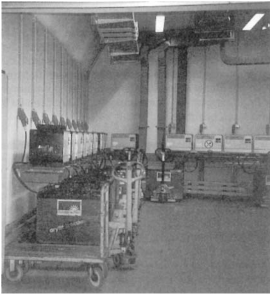
Figure 5.7 Charging station for batteries.
