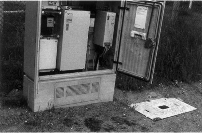
Figure 8.10 KVz cabinet with cable branch boxes.
