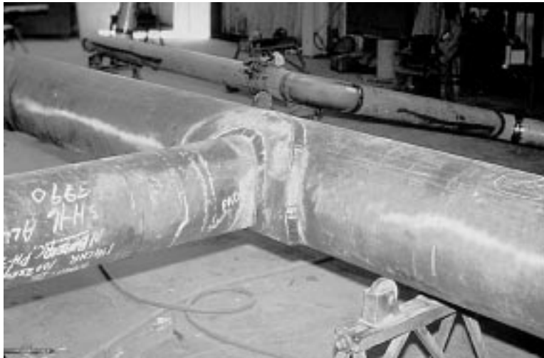
Figure 2.9 Pad reinforced branch connection.
