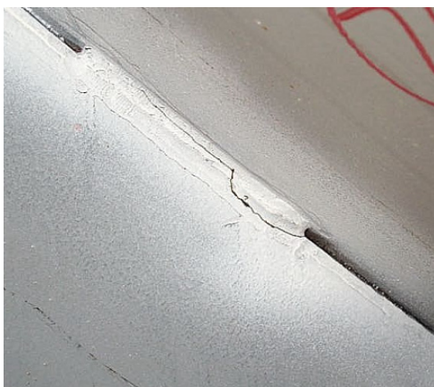
Figure 5.9 Crack found using magnetic particle inspection.
