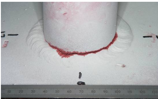
Figure 5.11 Crack found using dye penetrant inspection.
