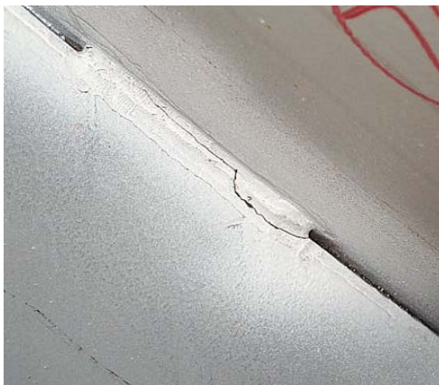
Figure 14.9 Crack found using magnetic particle inspection.
