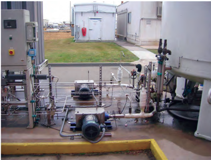
Fig. 4.14 Liquid nitrogen pump system with dual pumps (middle), liquid nitrogen tank (right), and controls and vaporizer (left). Courtesy of Air Products and Chemicals, Inc.
