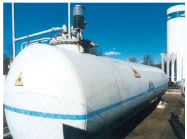
Figure 28: Methanol tank installation. The liquid nitrogen tank is seen in the background
