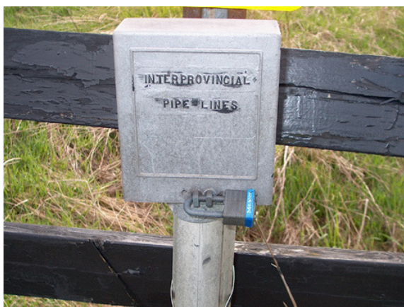
Figure 3-44: Lockable Test Station
