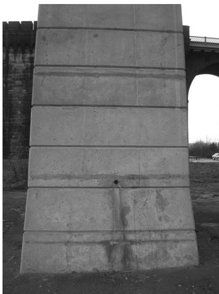
Figure 12.16 Egress of excess moisture.
