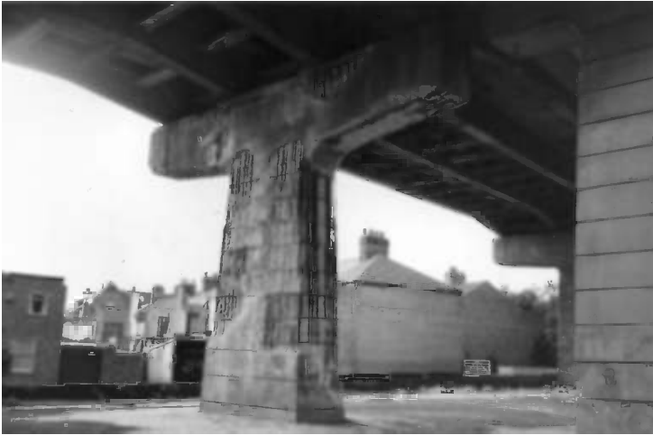
Figure 12.15 Deteriorated approach viaduct pier.
