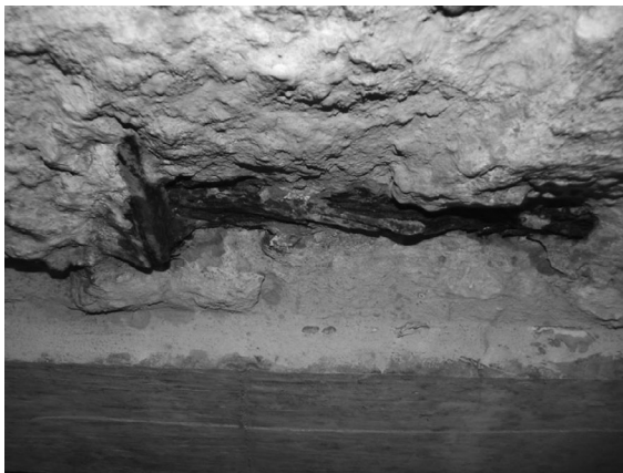
Figure 12.18 Corrosion of pre-stressing wires in precast beam.
