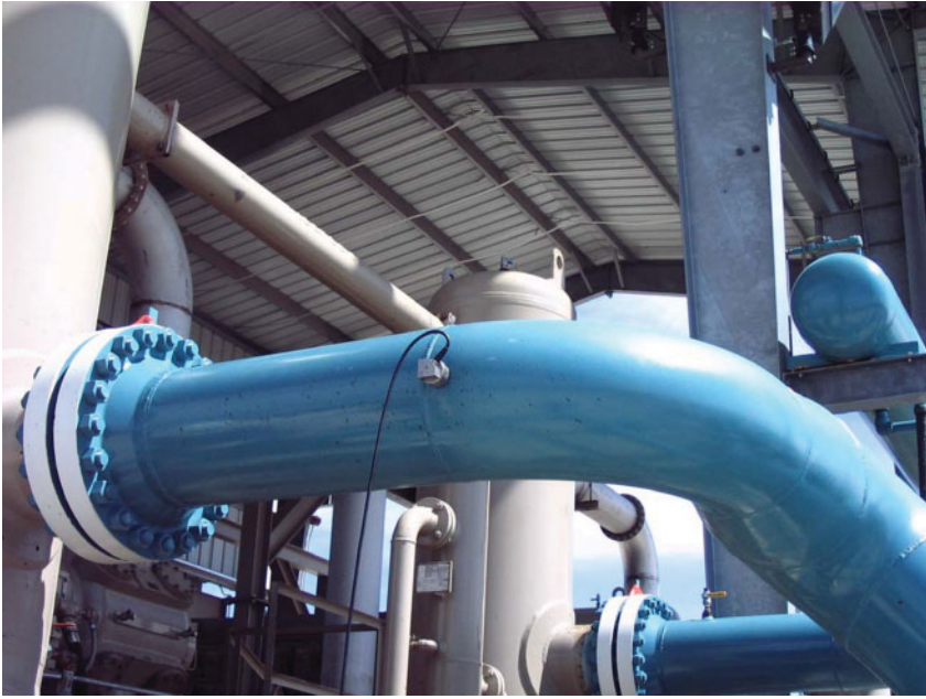
Figure 20.2 Mag-mounted tri-axial accelerometer on a pipe.
