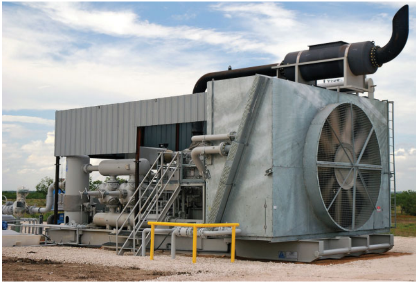
Figure 15.5 Reciprocating compressor driven by a natural gas engine.
