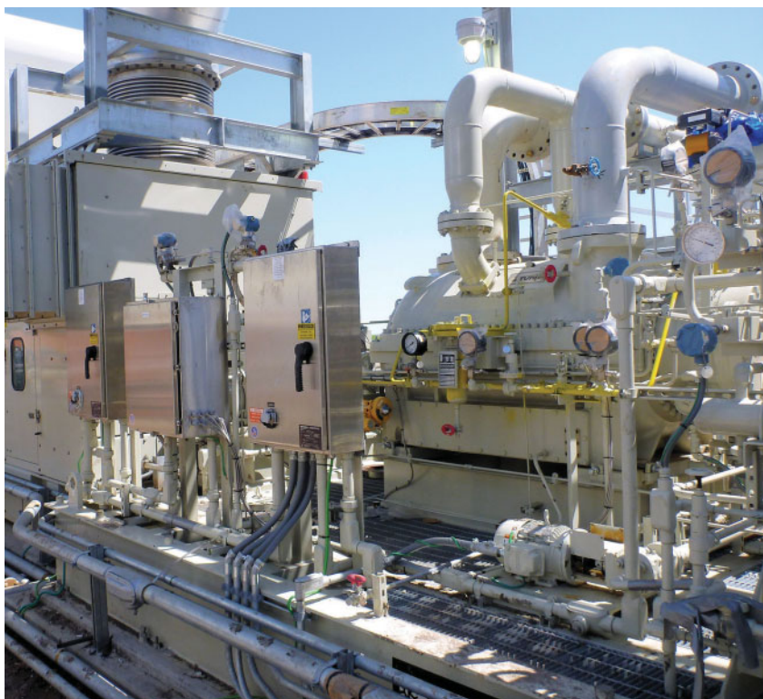
Figure 2.1 Centrifugal Compressor in a Petrochemical Facility.
