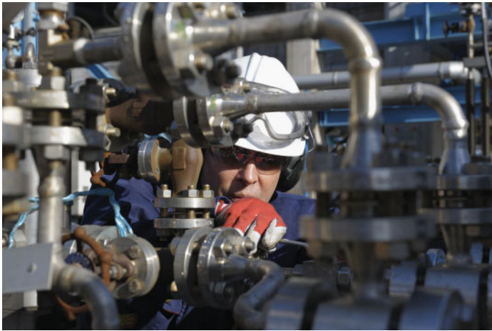
Figure 19.1 Operators must remain vigilant around reciprocating compressors and their associated piping. Poor designs and changing conditions can lead to excessive piping vibration.
