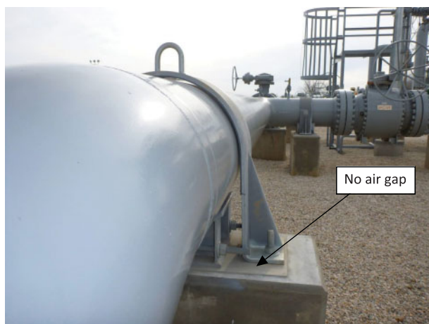
Figure 19.9 An incorrectly installed pipe clamp. Notice that with the clamp bottomed out there is an air gap between the pipe and the top of the clamp, i.e., there is no clamping force on the pipe.
