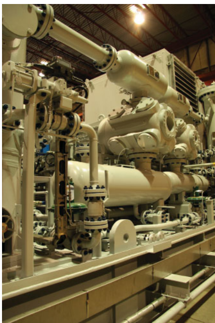
Figure 4.1 Skid mounted reciprocating compressor.
