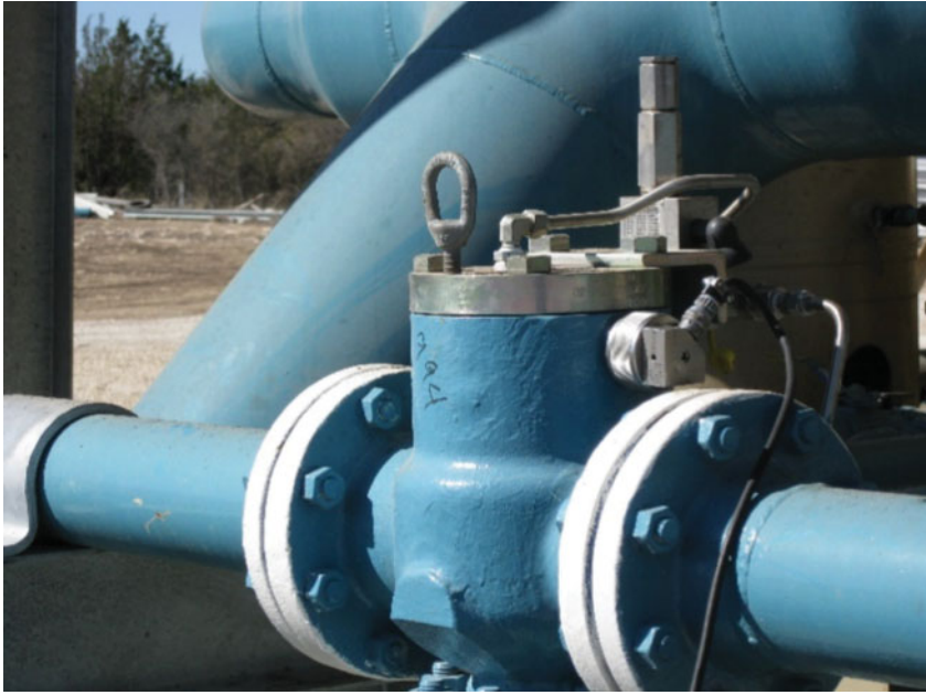
Figure 20.3 Mag-mounted tri-axial accelerometer on a valve.
