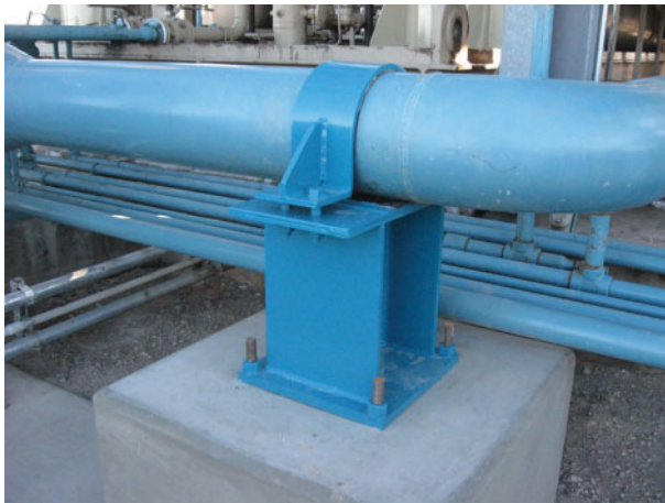
Figure 19.7 A properly installed pipe clamp bolted to a concrete pier. Notice that there is a gap between the pipe clamp and the pedestal support to ensure there is adequate clamping force present.
