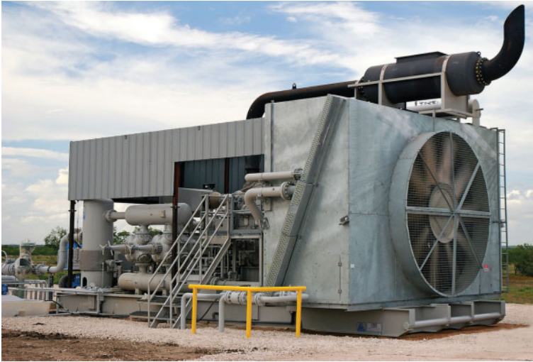
Figure 1.7 Air fin cooler, which is located on the far right of the skid, provides interstage cooling for the reciprocating compressor (far left).
