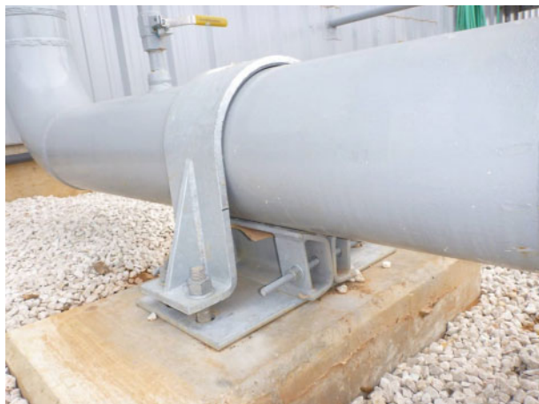
Figure 19.10 There is insufficient clamping force on this clamp due to the loss of wedge travel. (Notice that wedges are touching.).
