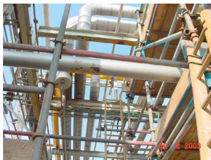
Isolated CUI in the center of a pipe
