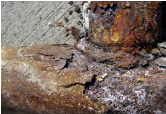
Figure I.1 Insulation removal highlighting corrosion product.
