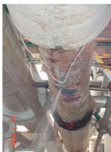
Localized CUI leading to metal perforation and leakage
