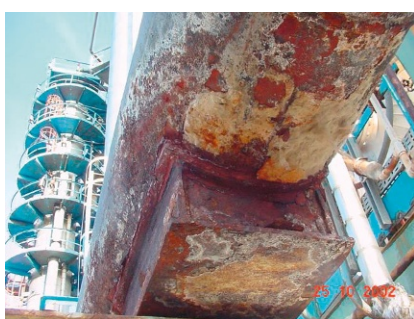
CUI at pipe support detail
