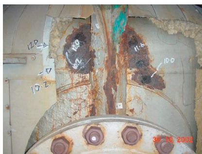
CUI adjacent to vessel manway
