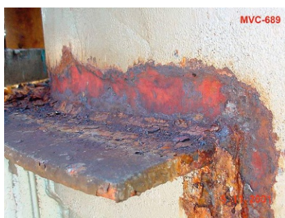
CUI at insulation support ring
