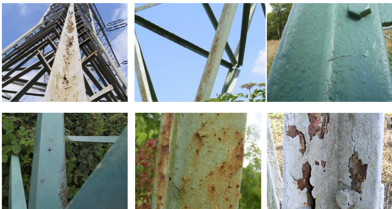
Fig. 11 Examples of failure of painting systems
