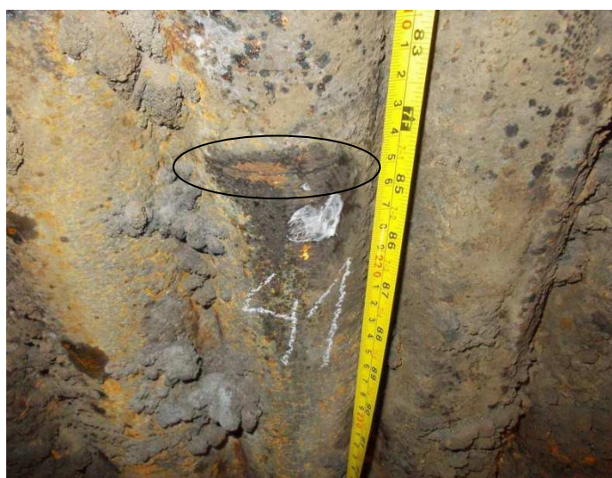
Fig. 1 Outer surface of pipe affected by flue gases.
